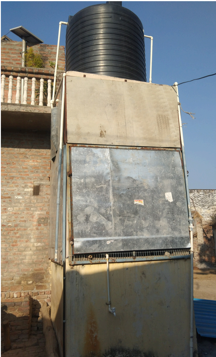
RO WATER FACILITY BAGHAU VILLAGE
